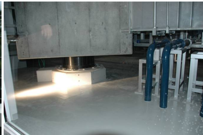
Quake-absorbing structure at data center
